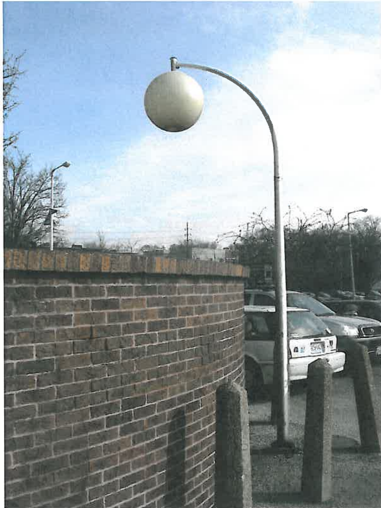
P10 – Parking Lot Light (Currently non-functional)
